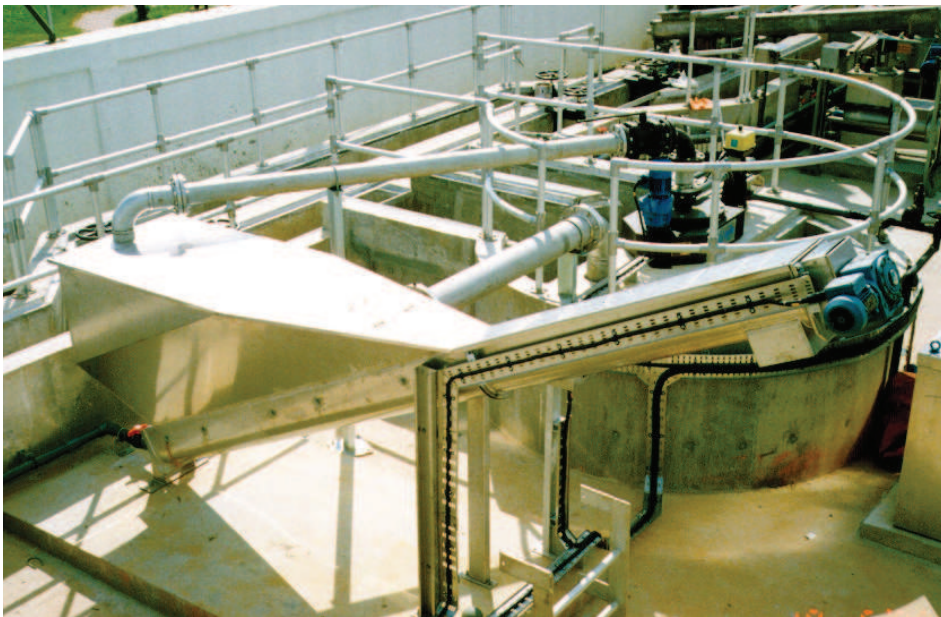
Typical grit classifier installation in wastewater treatment plant
